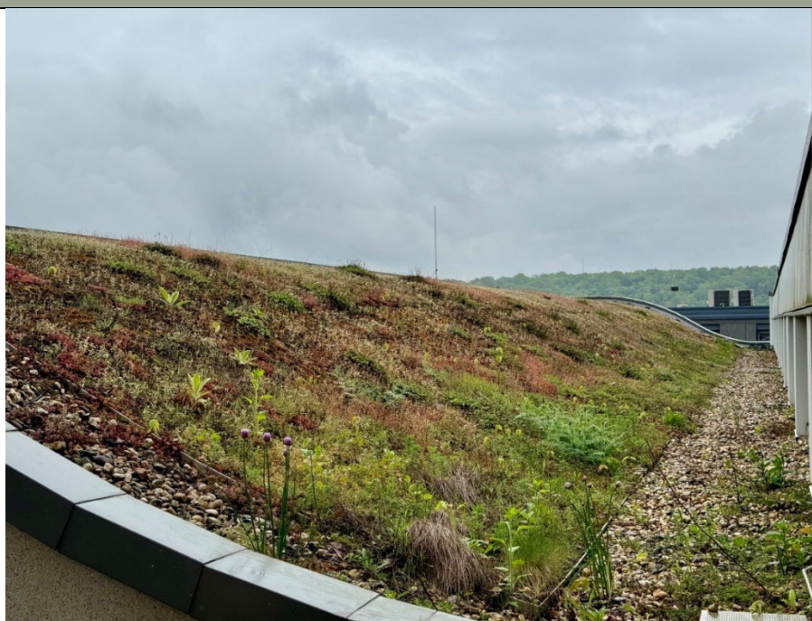
Figure 23: Green Roof of the Institute of Hydraulic Engineering and water management from the RWTH Aachen, ©Janine Lilia Freyer
